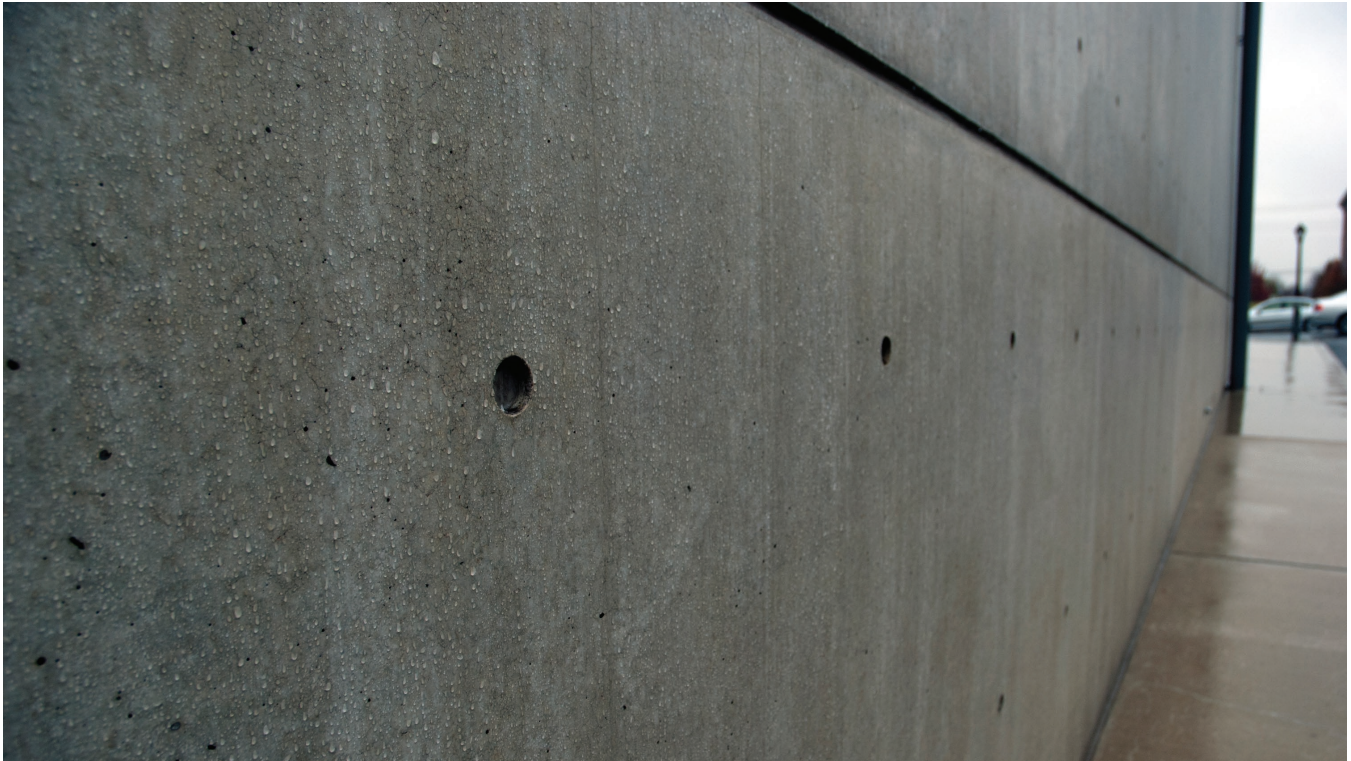
Figure 7. Pulitzer Arts Foundation, water being repelled by sealer. Copyright Liane Hancock.
